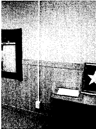
Interior and exterior surface-mounted conduits. (Johnson Consulting Engineers)
