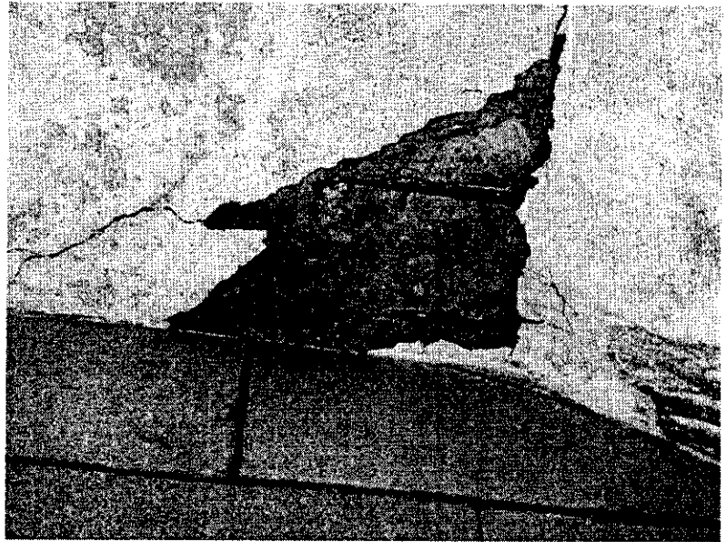
Exposed reinforcing steel in the soffit of the south stair landing. (Jaster-Quintanilla)
